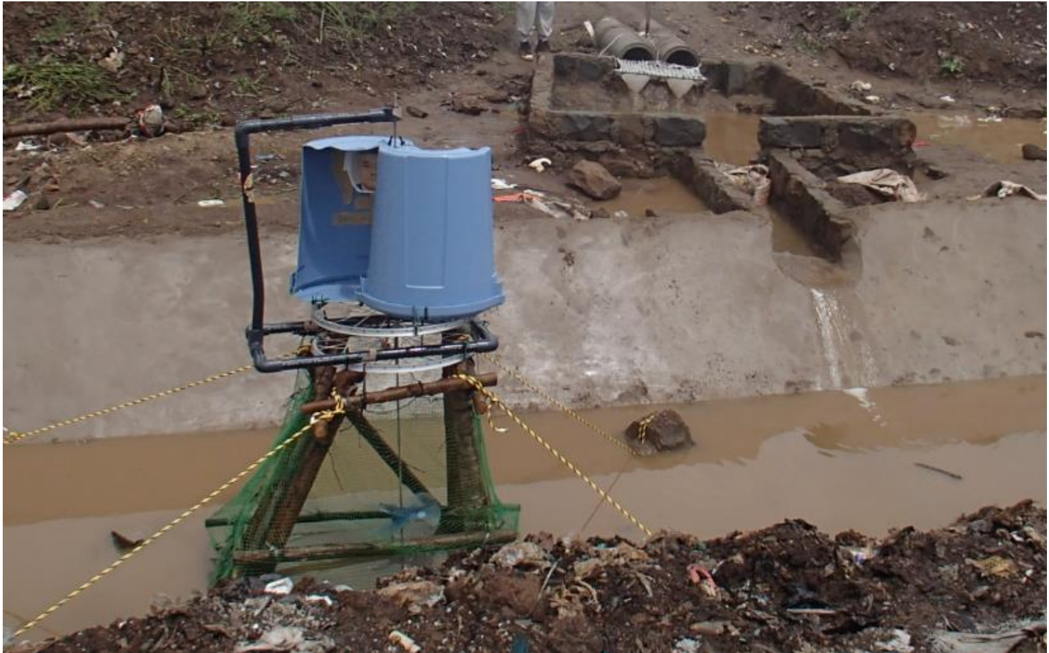
ECO-FAN: aeration system by natural air
